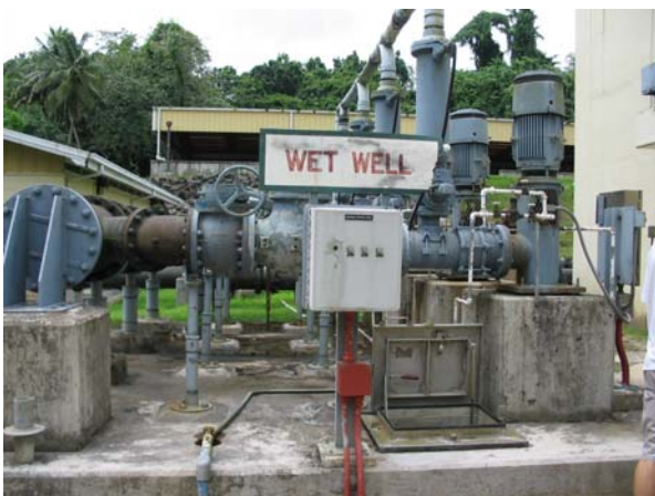
Water from the two sources is collected at the Wet Well.
