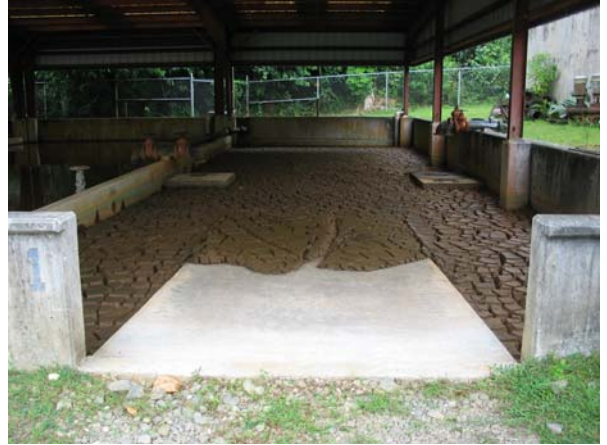
Sludge drying bed
